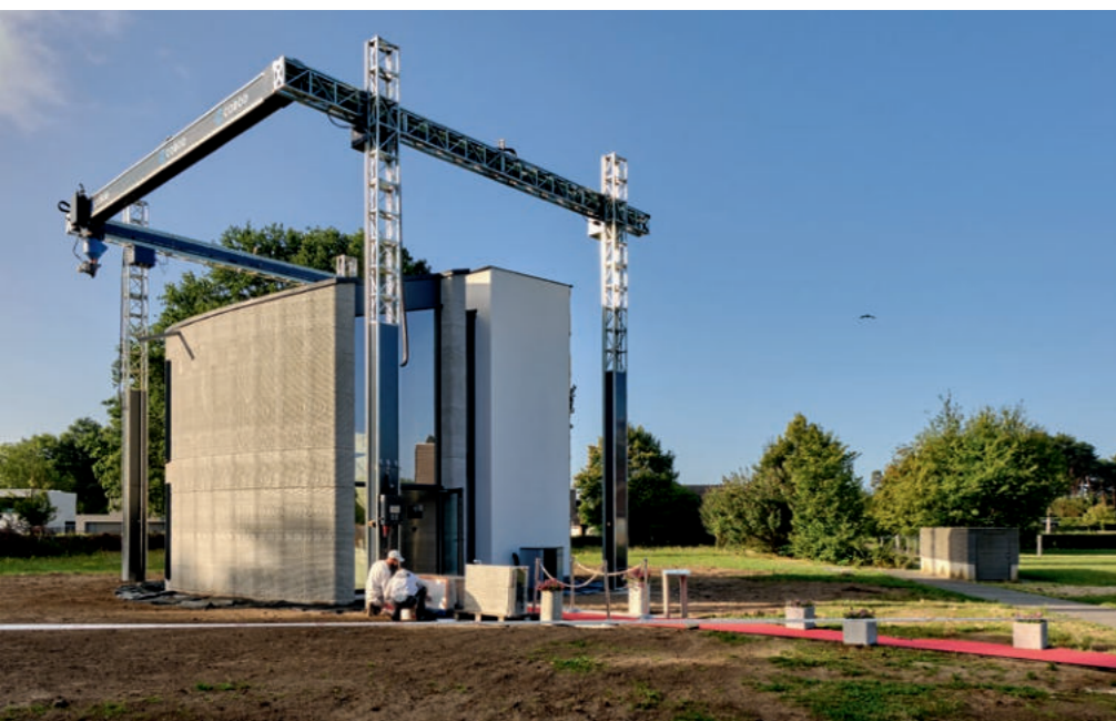
The residential/office building is located on Kamp C's premises in Westerlo, Belgium.
